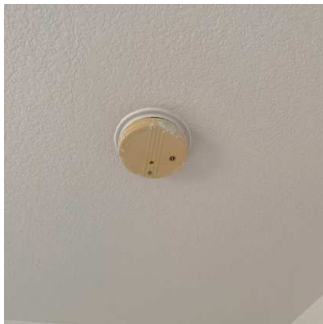
Smoke / CO detector 05/11/2020 5:30 PM
