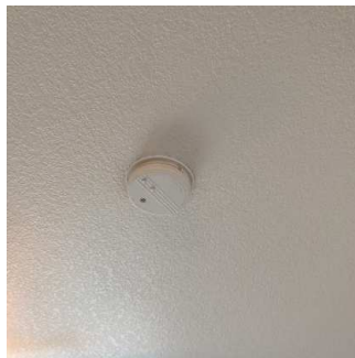
Smoke / CO detector 05/11/2020 5:21 PM
