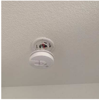
Smoke / CO detector 05/11/2020 5:16 PM
