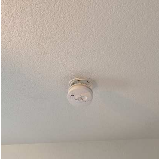
Smoke / CO detector 05/11/2020 5:27 PM
